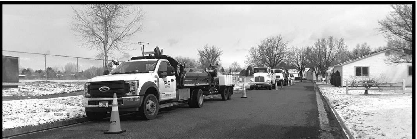
A crew and vehicles from Primoris Services Corp. of Minnesota work to run a fiber optic cable underground up the west side of the Vineyard.
